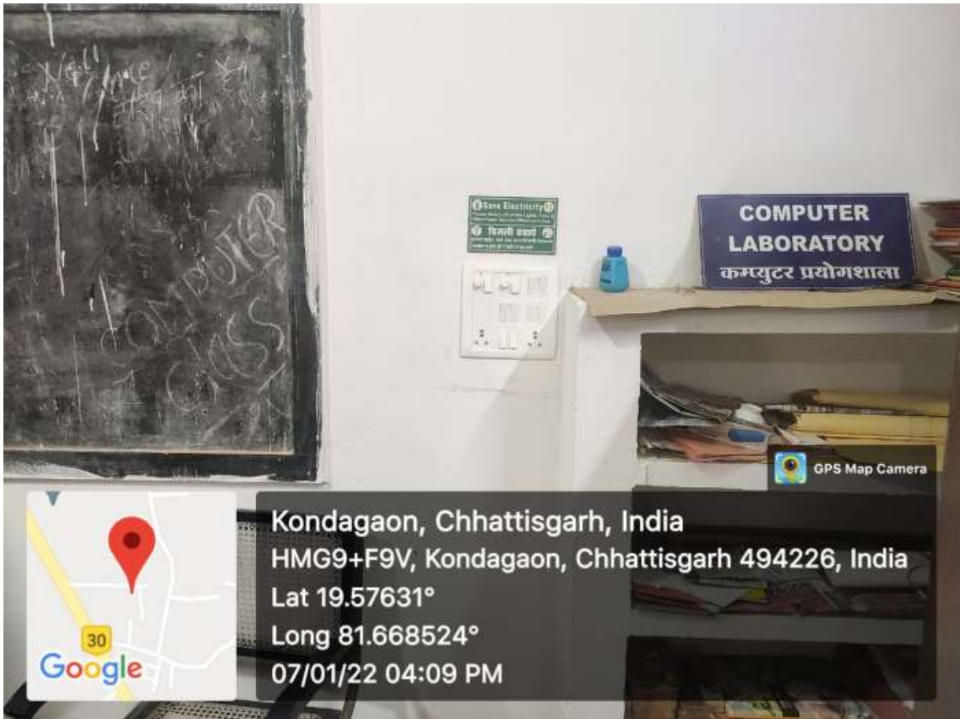
Fig.: “Save Electricity” message on switch board.
